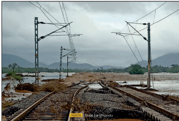
Photo 4: Tracks Washed Away in Guntakal – Tirupati flood – Many trains diverted Or Cancelled
